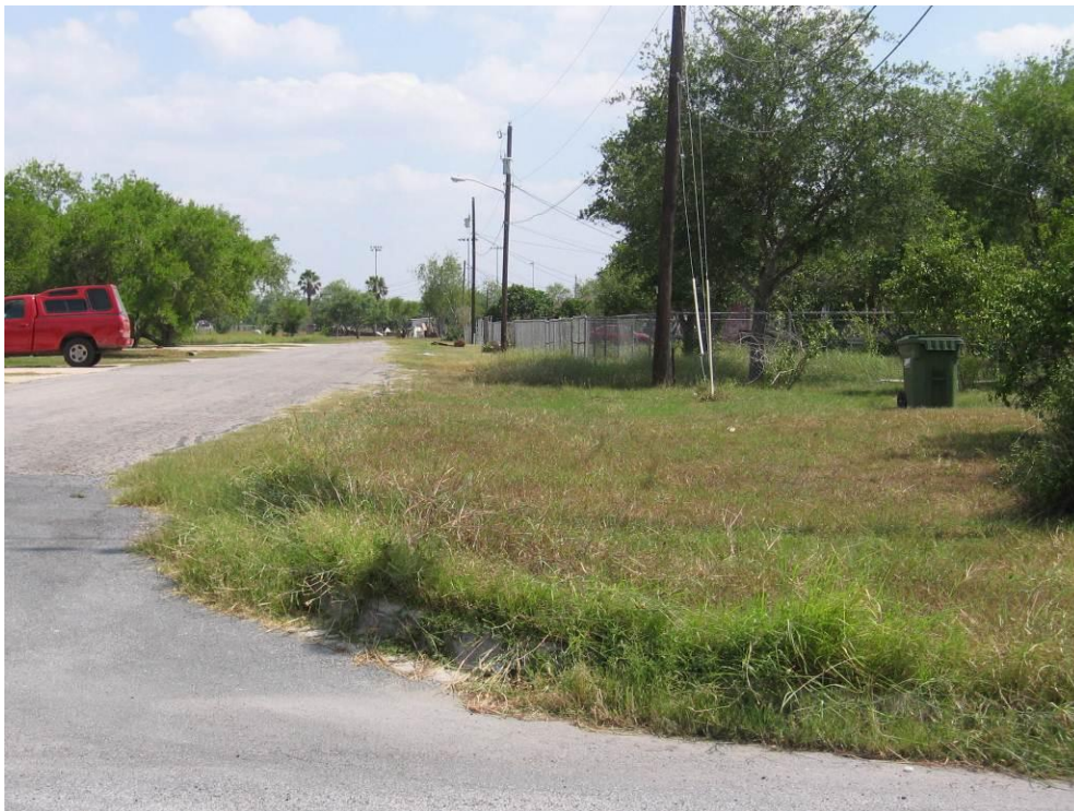
Figure 7B. Roadside ditch within residential area in poor condition
