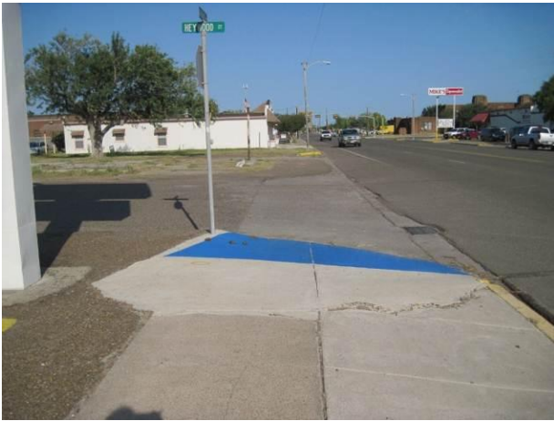
ADA ramps on Harrolds Street. Ramps are present but not always in standard condition.
